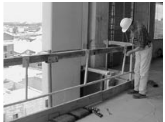
Figure 8 Temporary guardrail used to replace mesh to enable work to take place on the curtain wall securing bolts
