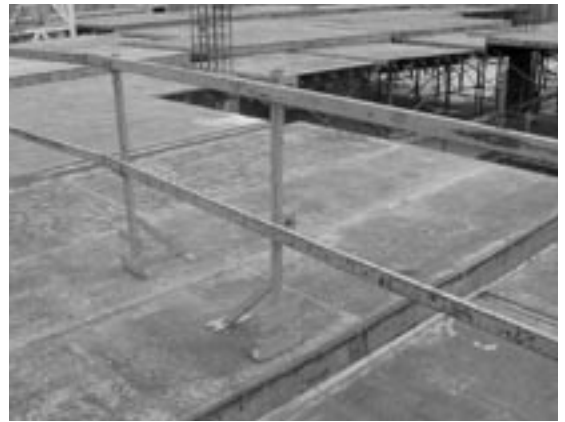
Figure 20 Table form guardrails set back a safe distance from the open edge
