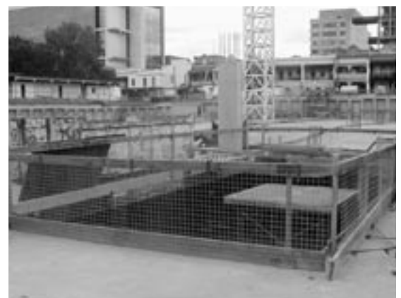
Figure 1 Guardrails protecting an open penetration through the slab
