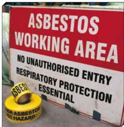
Figure 2: A warning sign informing people of asbestos work in the area.
