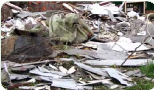
Broken asbestos cement materials from a demolition
